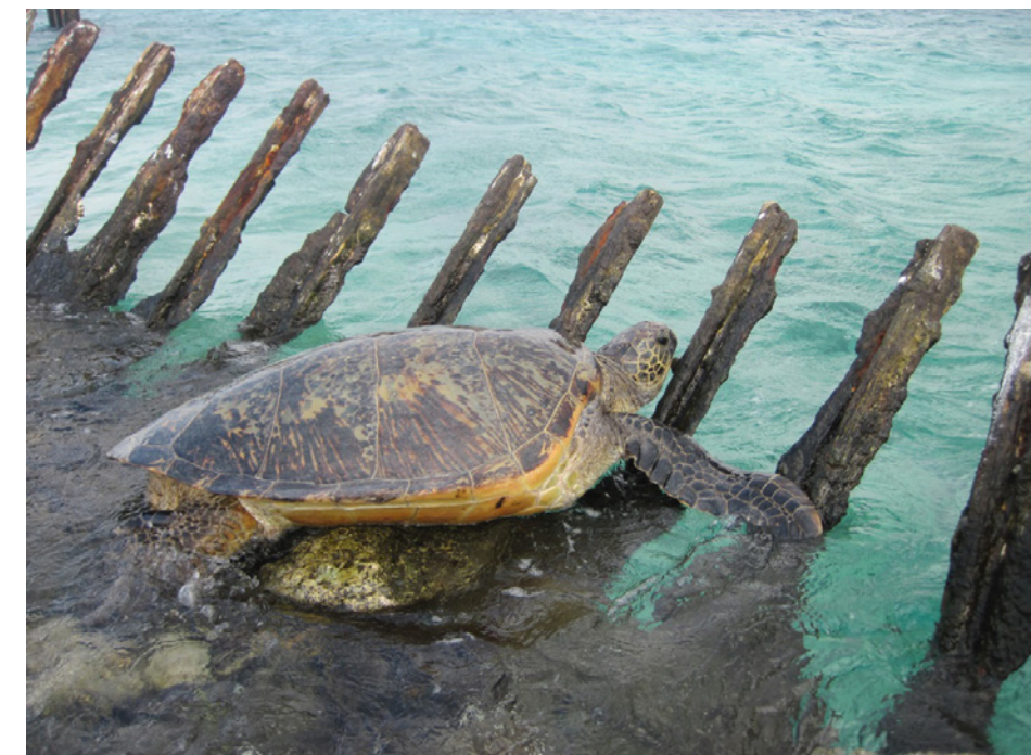
LEFT One of nine female honu that became entrapped in Tern's degraded seawall in recent years. She was released back into Monument waters without incident, but with the island unstaffed now and in the future, similarly entrapped turtles will likely perish. Photo by USFWS
