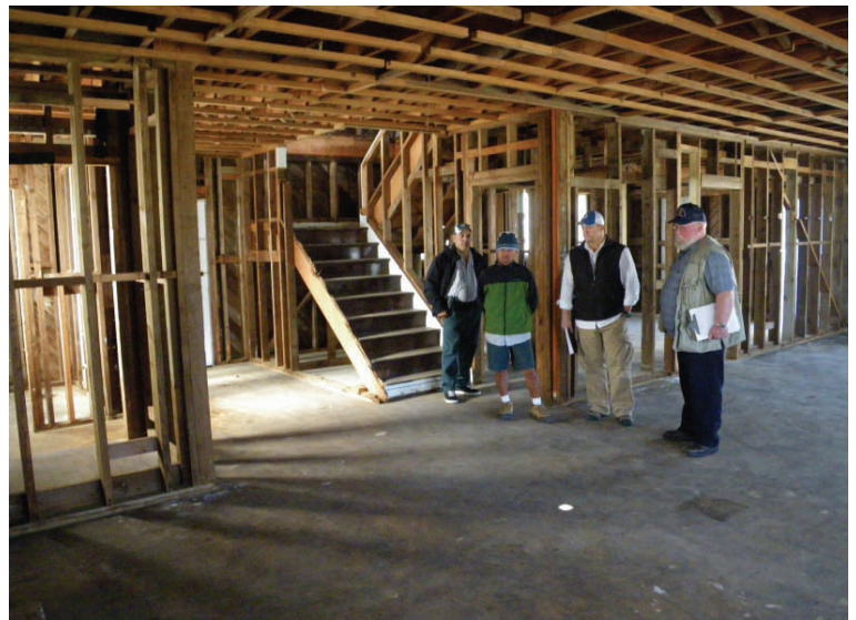
Historic officer's home fully gutted of asbestos and lead paint, and ready for energy-efficient renovations.
