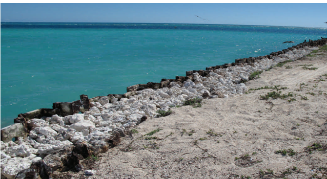
Filling in the gap between corrugated metal sheets of the old seawall prevents wildlife from becoming entrapped.
